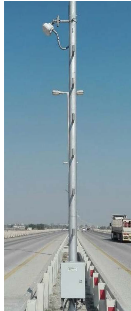
Fig. 1: DATACAR System portable installation including Traffic Radar Sensor and METEODATA unit
