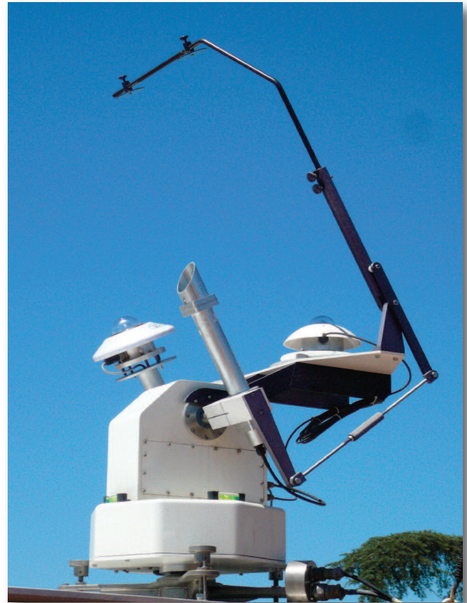
Meteorological Station with SunTracker-3000
