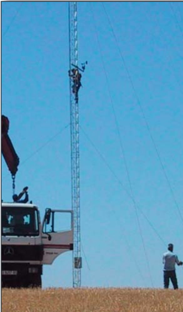
Mounting the wind sensors and the Data Logger / Transmitter, on a 60-meter stainless steel meteorological tower
