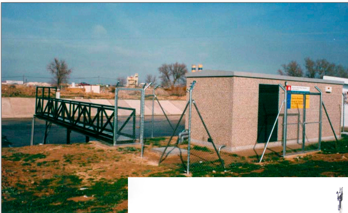
Up: General view of a riverside analyzer's housing
